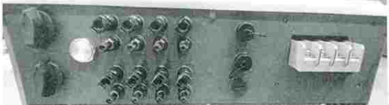
DC SWITCHES, PV CONNECTORS, WIFI/GPRS AND AC TERMINAL BLOCK
